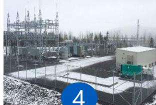
4 Project substation (grid tie)
